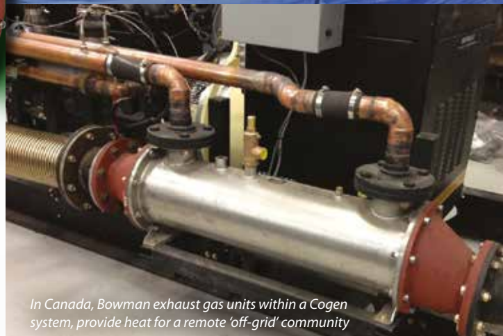
Bowman exhaust gas units are installed in the CHP system within the British Arctic Survey's Halley VI research station
